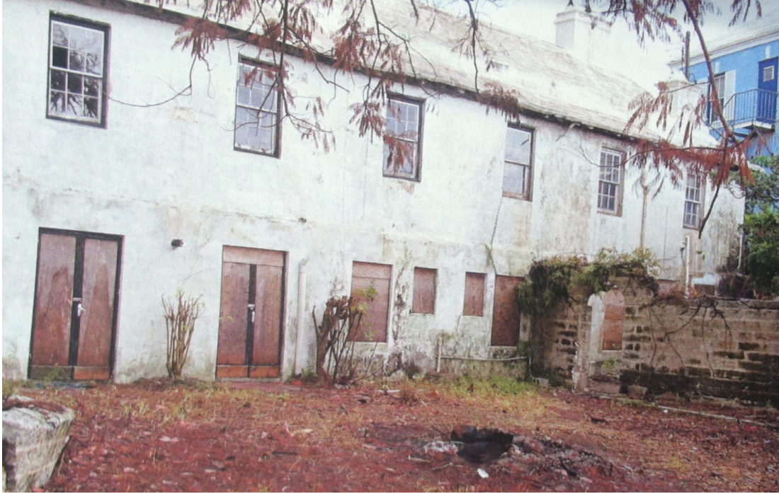
Figure 1.6: Queen of the East's southern elevation overlooks Hamilton Harbor. The twentieth-century addition is at far right. Courtesy Bermuda Department of Planning, 2008.
